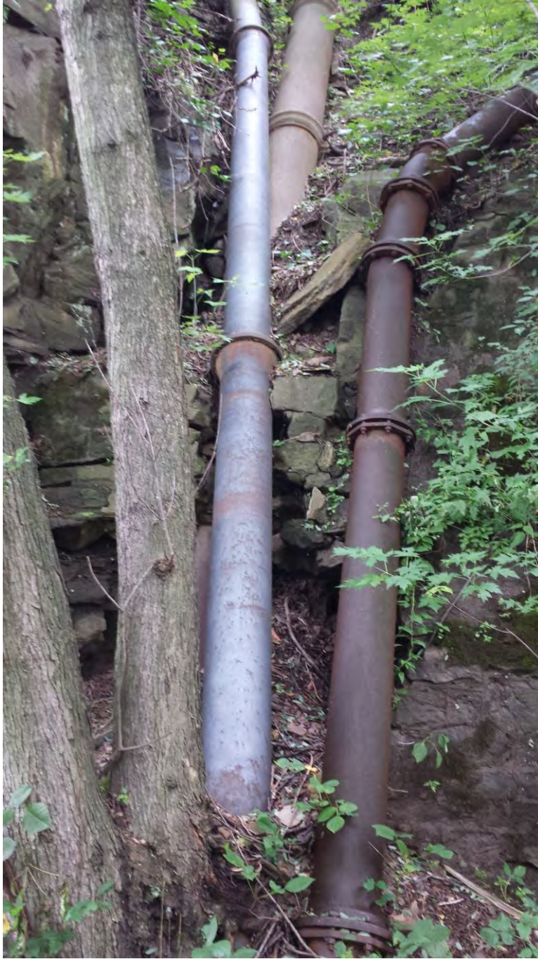
View looking up hillside toward tank from west side of pipe bridge
