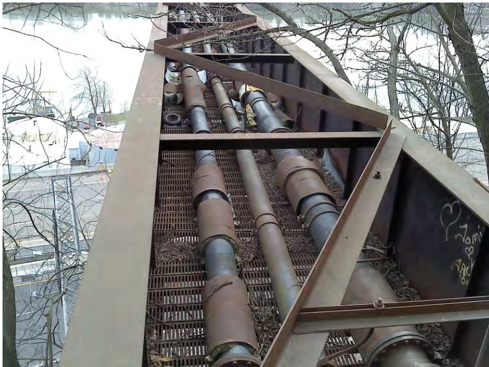
View looking at piping across pipe bridge from west side
