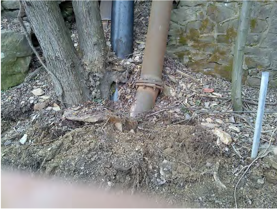
View looking at bottom of hillside from west side of pipe bridge
