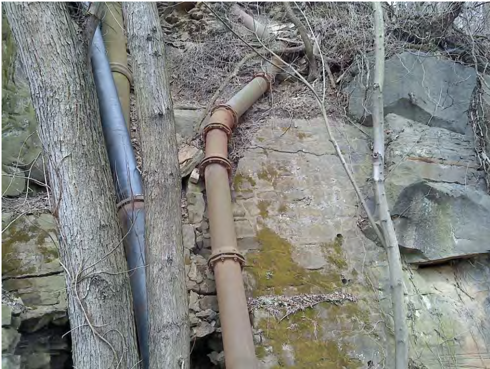
View looking up hillside toward tank from west side of pipe bridge
